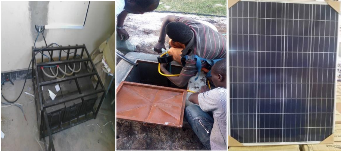
Water pump system and installation of tanks
