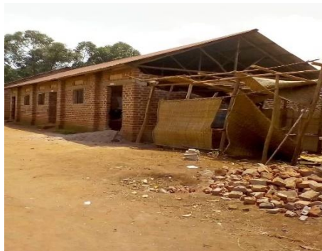
Classroom Shade and Originally collapsed Pin Wall
